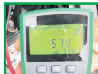
Battery status test
